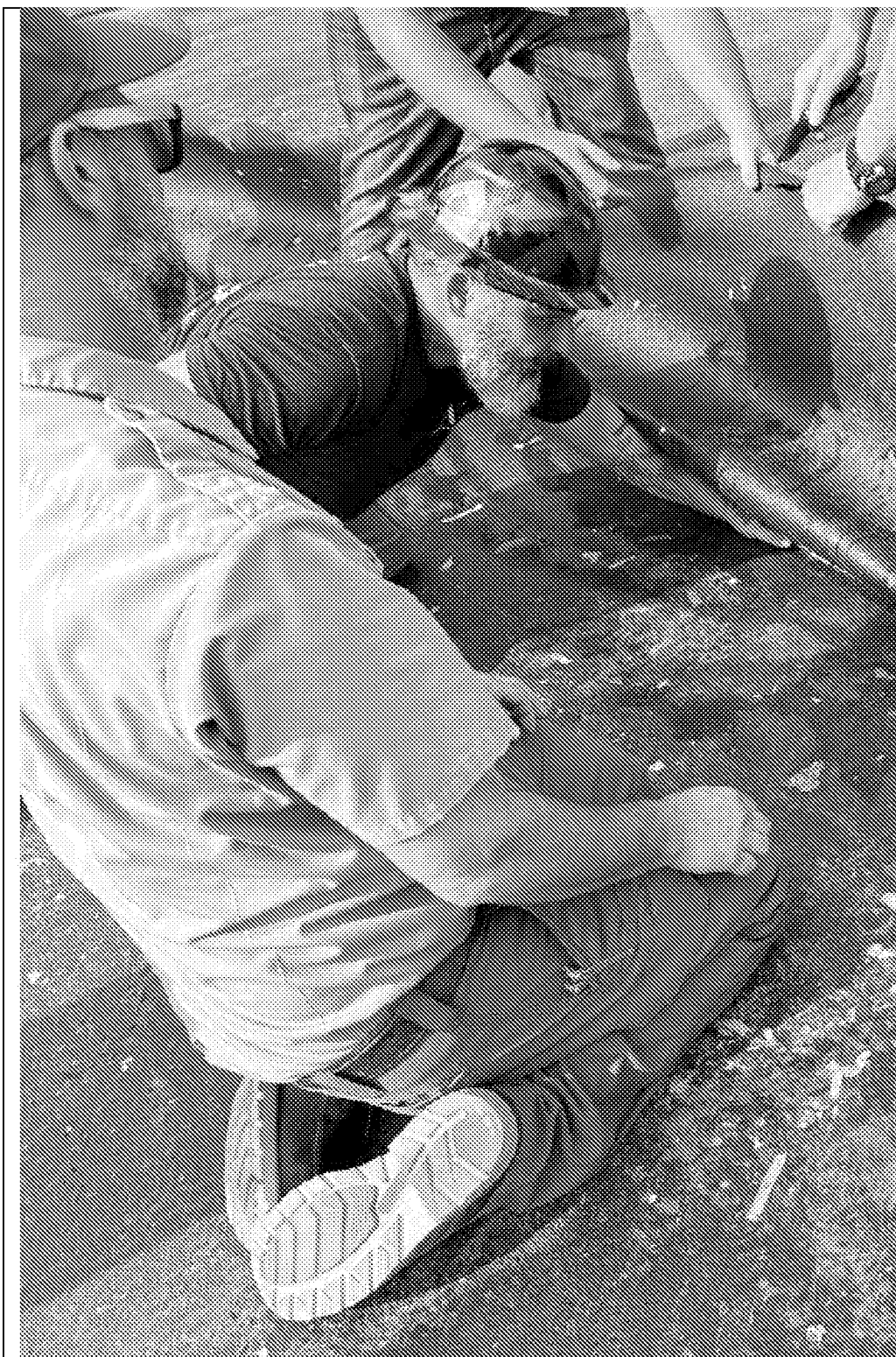
Photo #5 – Examination of delaminated coating at tranverse expansion joint between Bays 04 and 06
